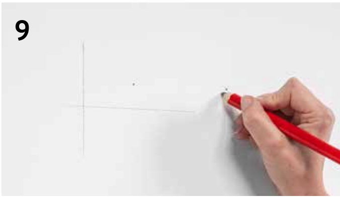
9 Use a pencil to mark the first drilling point on the wall
